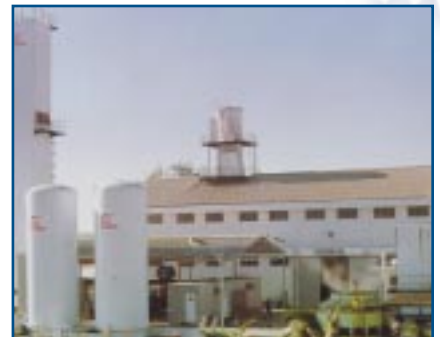
Cosmodyne’s ASPEN 1000 air separation plant was originally installed at the BOC Pakistan’s facility in Hub, Pakistan (shown here). After 18 months of service at this location, the plant was transported 800 km (500 miles) northeast to Lahore where it currently operates.
