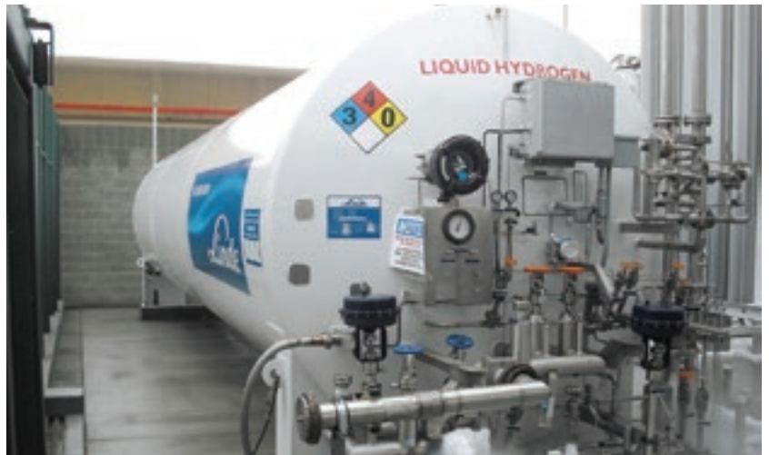
Hydrogen sub-cooler with VJ piping and heat exchanger designed to increase efficiencies when pumping
