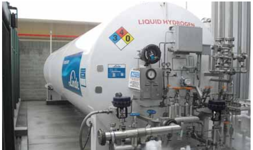
Hydrogen sub-cooler with VJ piping and heat exchanger designed to increase efficiencies when pumping
