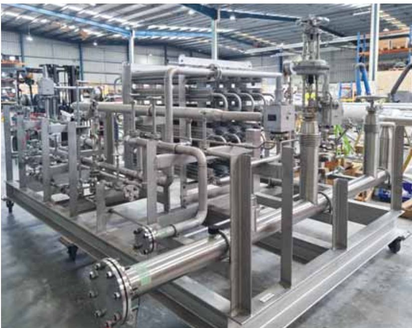
LH 2 Loading skid for Liquefaction Plant to Tanker Transfer
