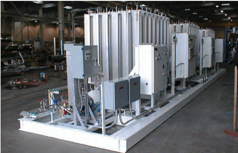
Skidded high pressure ambient vaporizer system
