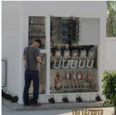
COLD BOX GROUND LEVEL VALVES AND INSTRUMENT VALVES
