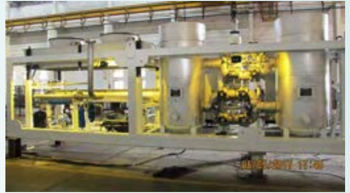
TSA DRYER CONTROL VALVES lighting included pre-installed on all skids-
