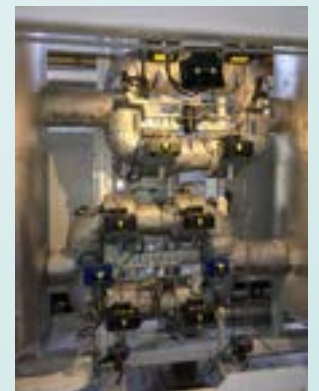
ADSORBER BED VALVES WITH SOFT INSULATION
