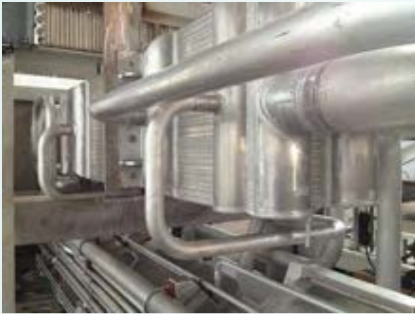
BRAZED AL HEAT EXCHANGER AND PIPING
