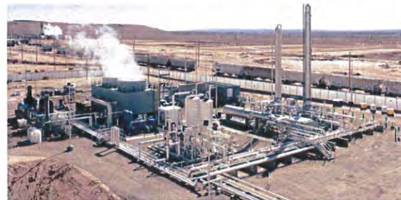
Figure 3. Gas treatment system.
