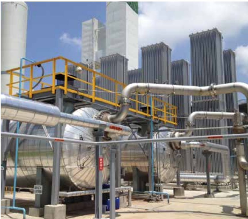
Water bath vaporizers with ambient air vaporizer backup option
