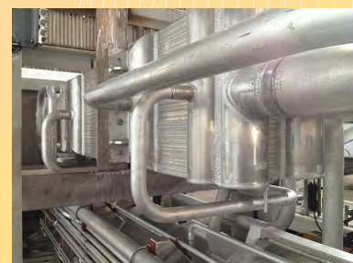
BRAZED AL HEAT EXCHANGER AND PIPING
